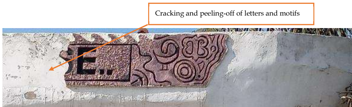
Figure 2: cracking and peeling-off relief sculpture lettering and motifs, Komanste, Mfatsiman District. Anonymous, n.d.. copyright 2019 by James Ekow Appiah. Photograph with permission.
