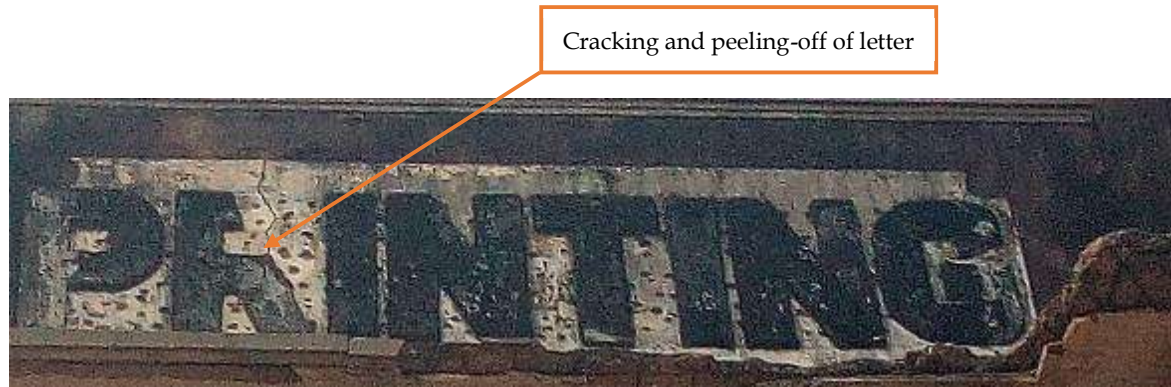
Figure 1: Cracking and peeling-off relief sculpture lettering, Prospect lodge, Cape Coast. Anonymous, n.d.. copyright 2015 by James Ekow Appiah. Photograph with permission.
